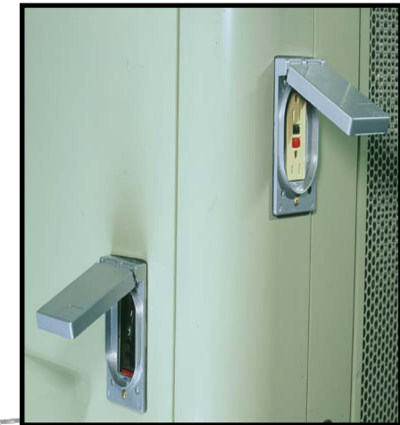
Disconnect Switch 115VAC Outlet
